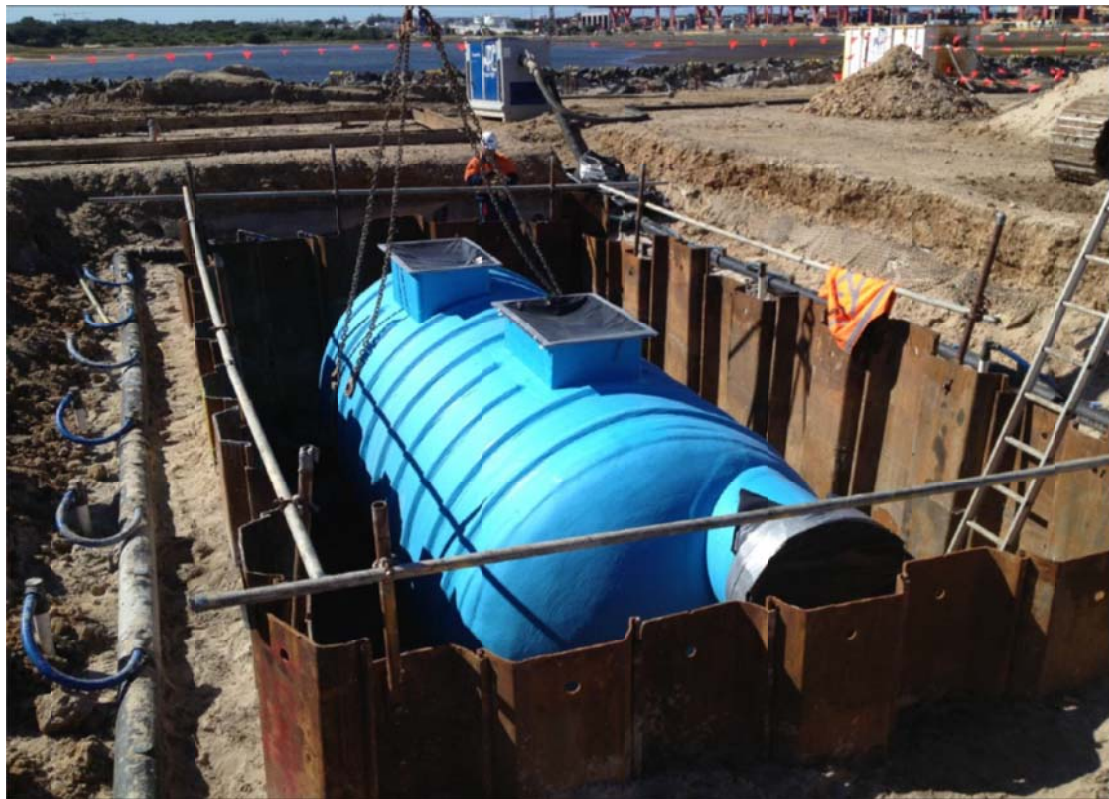
Figure 5 A SPEL Environmental ‘Stormceptor’ separator unit being installed during construction of the SICTL Terminal in 2013.
